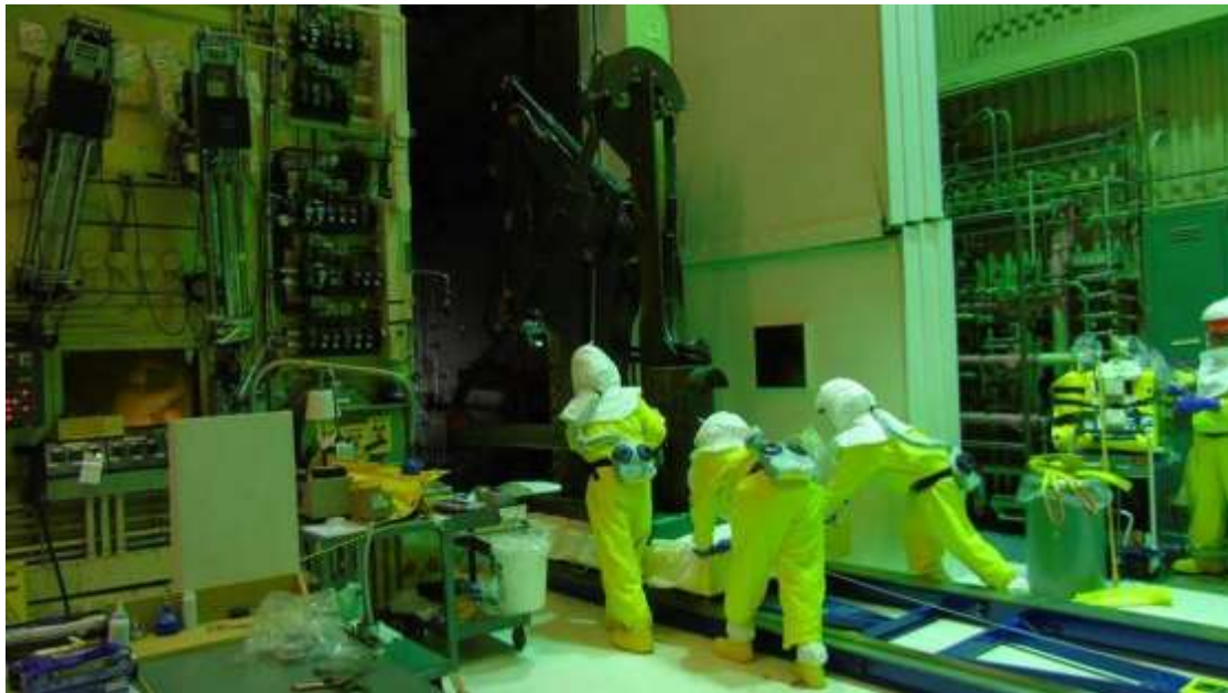
Workers at Hanford have been preparing to clean up a highly radioactive spill under the 324 Building for six years. The spill's contamination recently was discovered to be significantly larger than expected. Courtesy Department of Energy
