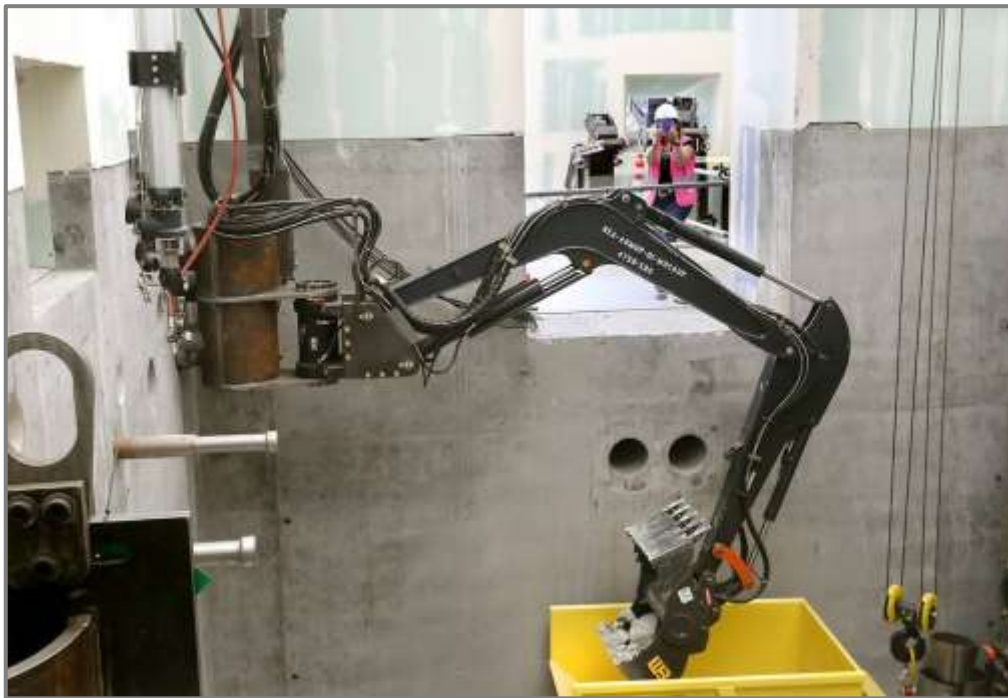
Workers have been practicing using remote-operated equipment at a mock-up of the 324 Building to prepare to dig up highly radioactive waste. Bob Brawdy Tri-City Herald file
