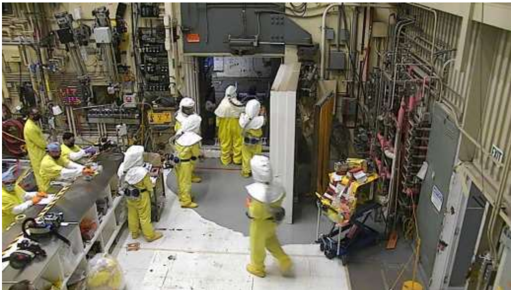
Workers started preparing to clean up a highly radioactive spill beneath the Hanford site 324 Building near Richland and the Columbia River in 2017. The spill was recently found to be much larger than expected. Courtesy Department of Energy
